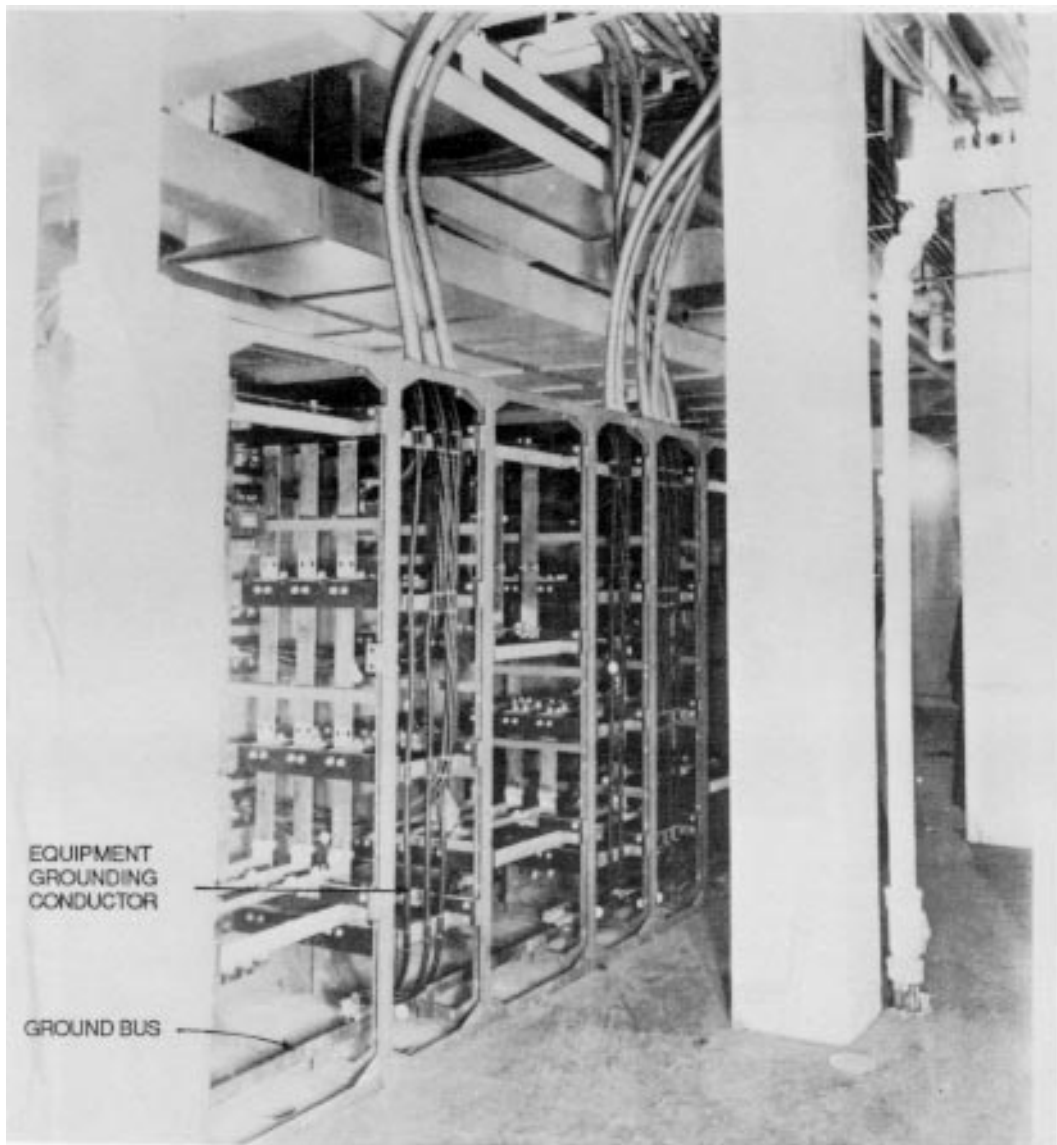
Figure 45—Indoor Unit Substation — Back View Showing Use of an Independent Grounding Conductor with Each Circuit
