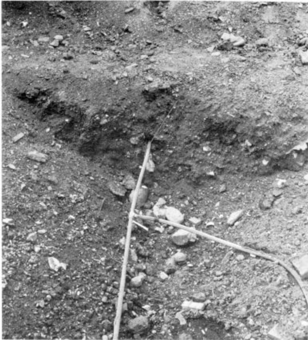
Figure 38—Thermal-Weld Junction in Underground Grounding Conductor
